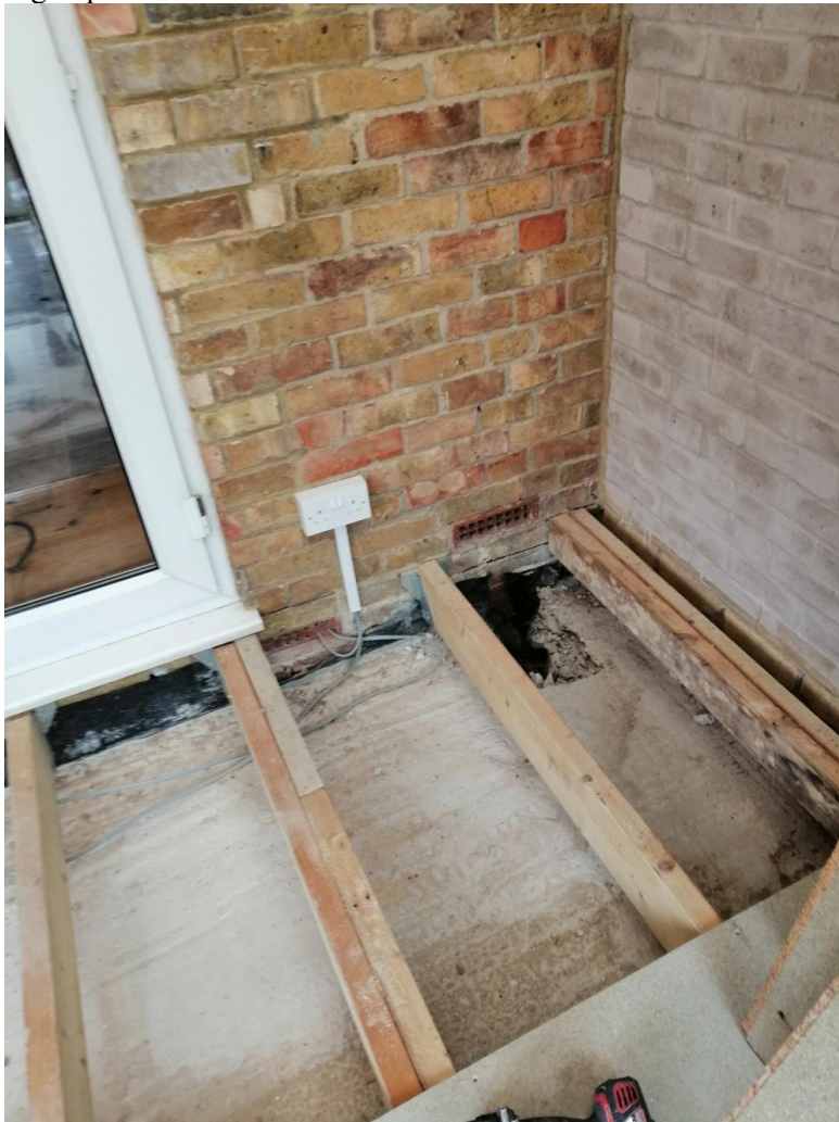
Fig 6 Old conservatory the floor beneath the wooden beams is concrete over a membrane and this showed no sign of water ingress. The trial pit holes showed the water table height
