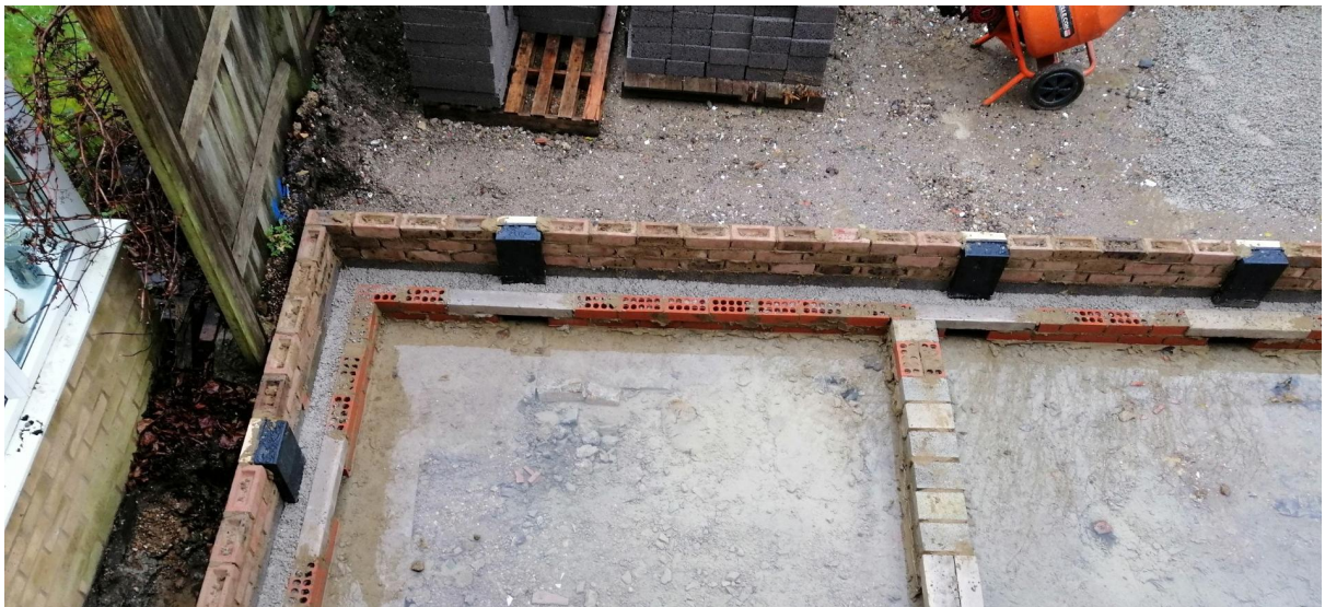
Fig 4 – water on inside but not outside.
