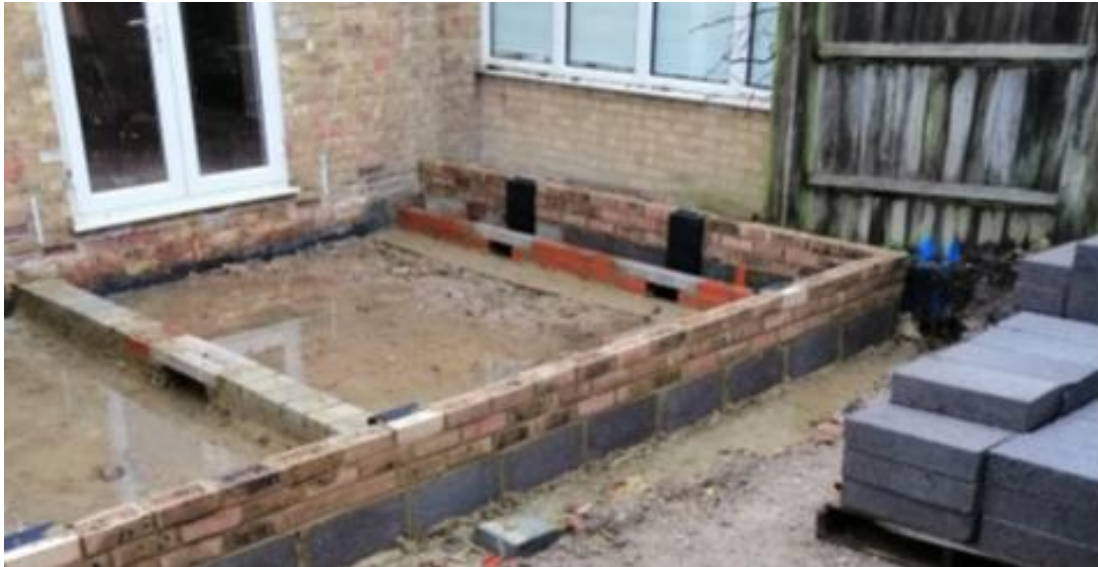
Fig 5 previous week water on inside but not on outside.
