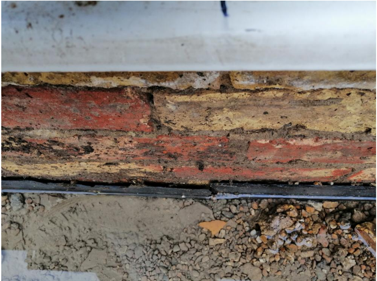
Fig 3 Existing DPC under dining area in the original house
