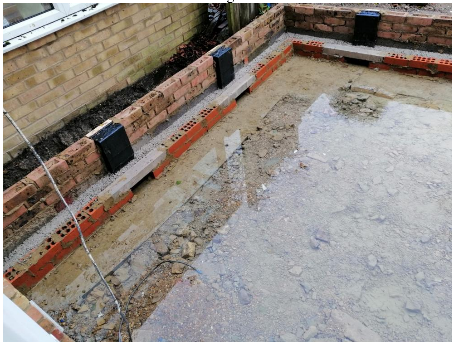
Fig 2 Cavity is dry but the extension has water – is this surface water or water table?
